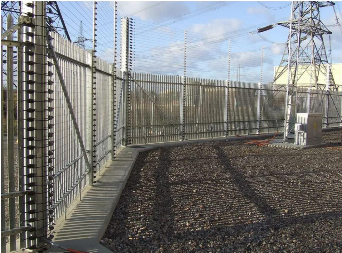
Plate 4.5 Typical examples of high security external fencing
