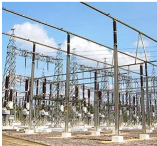
Plate 3.1 Typical AIS external switchgear (400kV single busbar)
